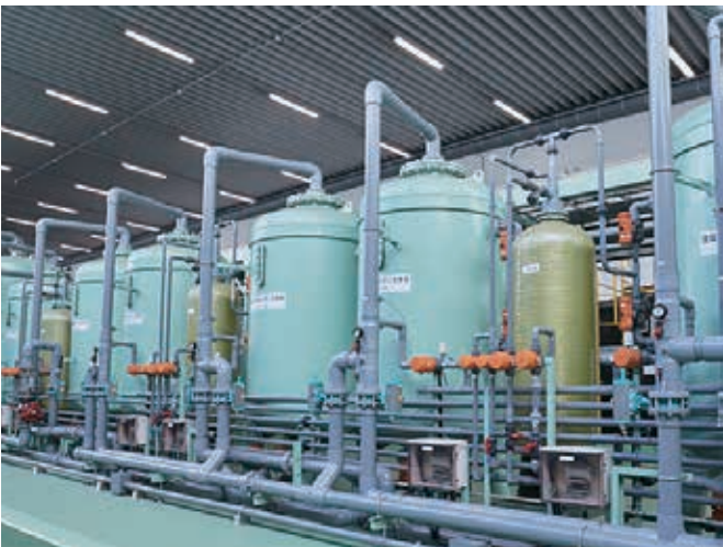
Conserving water - manufacturing
